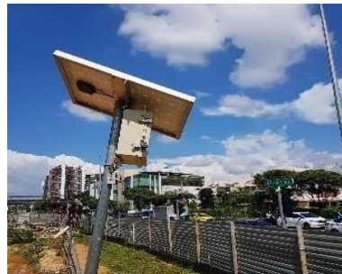
Solar source for our noise monitoring system
