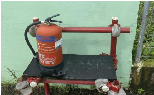
Recycle GI Pipe for fire extinguisher stand
